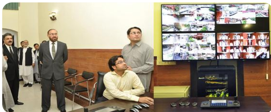
‘CCTV Control Room’
